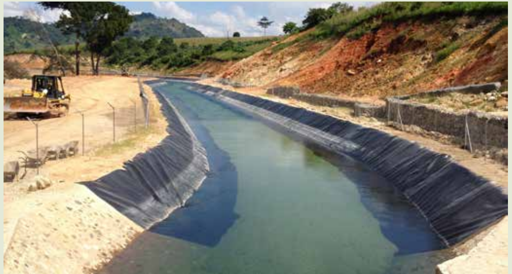
Pungwe C Hydro power
